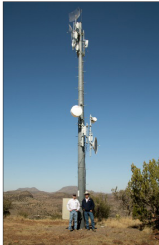
Tower with backhaul and Access Points
